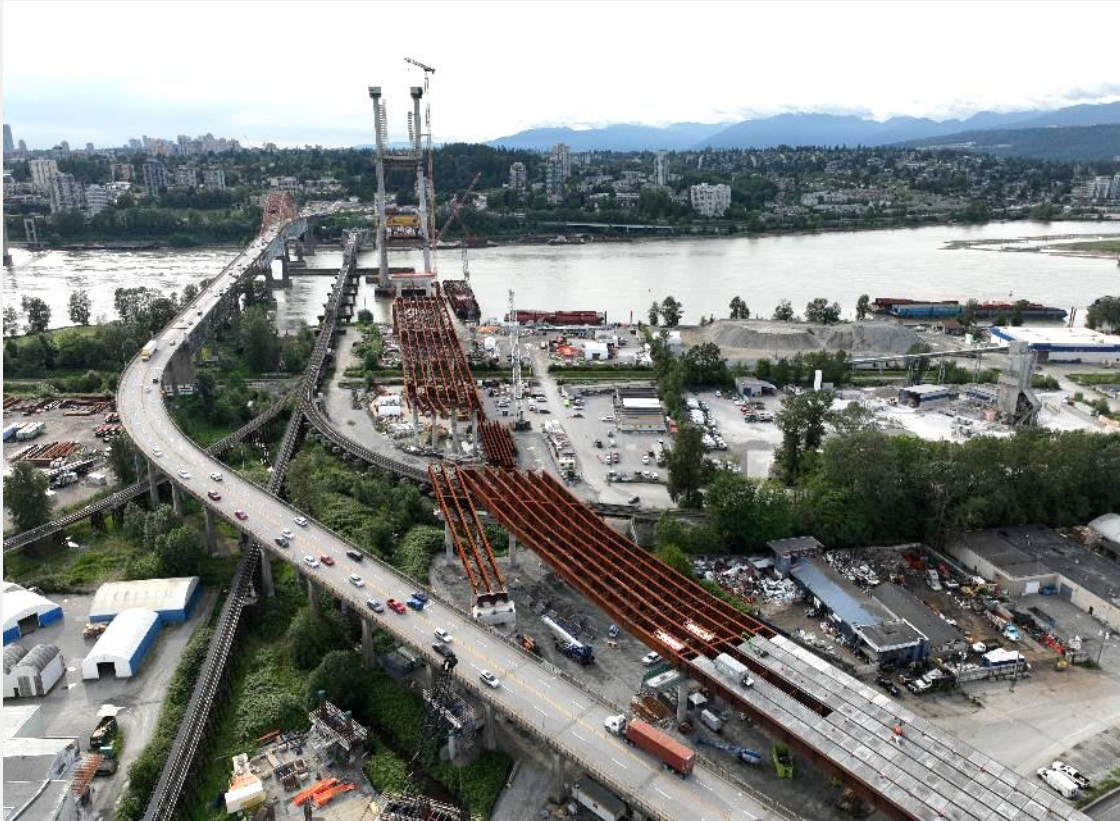
Photo 3: Looking northeast towards Pier S1 – South approach girder and deck installation works ongoing
