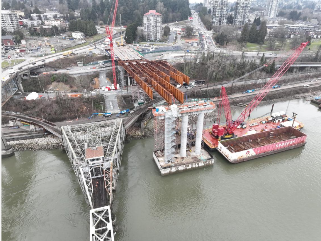
Photo 5: Barge and crane positioning next to N1 Tower to support girder installation
