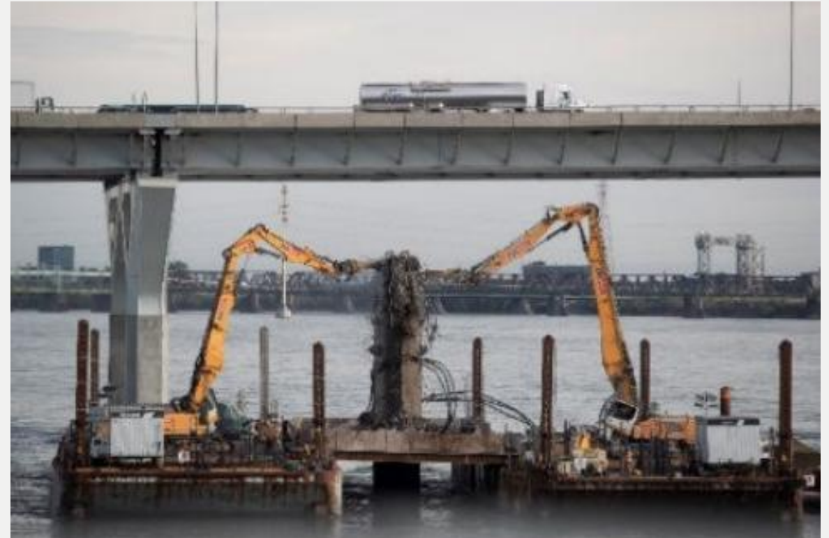
Photo 8: Example photo showing deconstruction of the original Champlain Bridge in Montreal, Quebec
